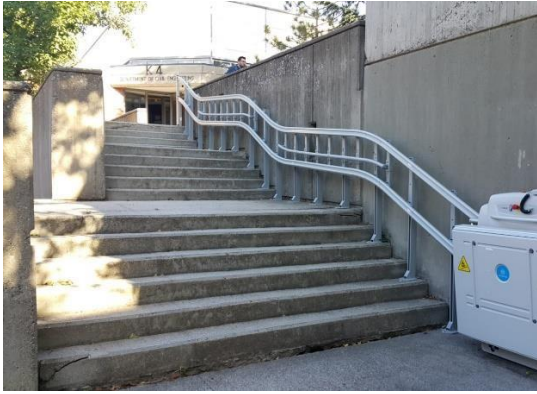
platform lifts for disabled
