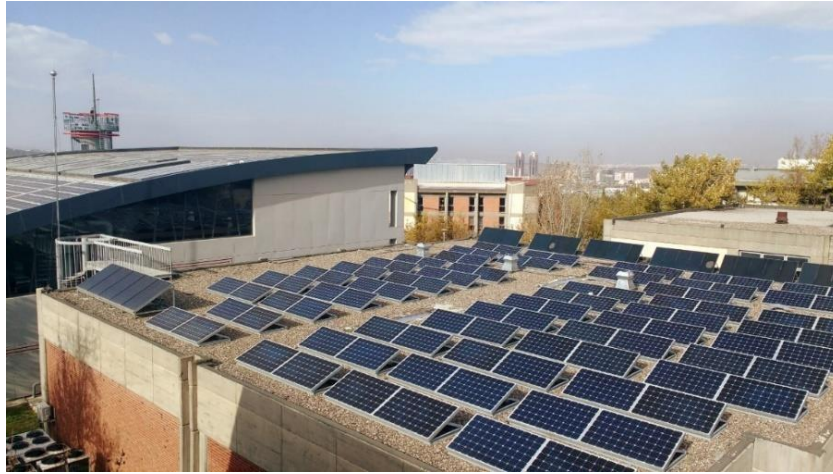
Solar Panel (METU Department of Electrical and Electronics Engineering Building)
